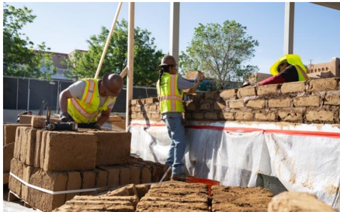
Adobe bricks are placed within a steel frame by Avanyu General Contracting at the site of the New O’Keeffe.
